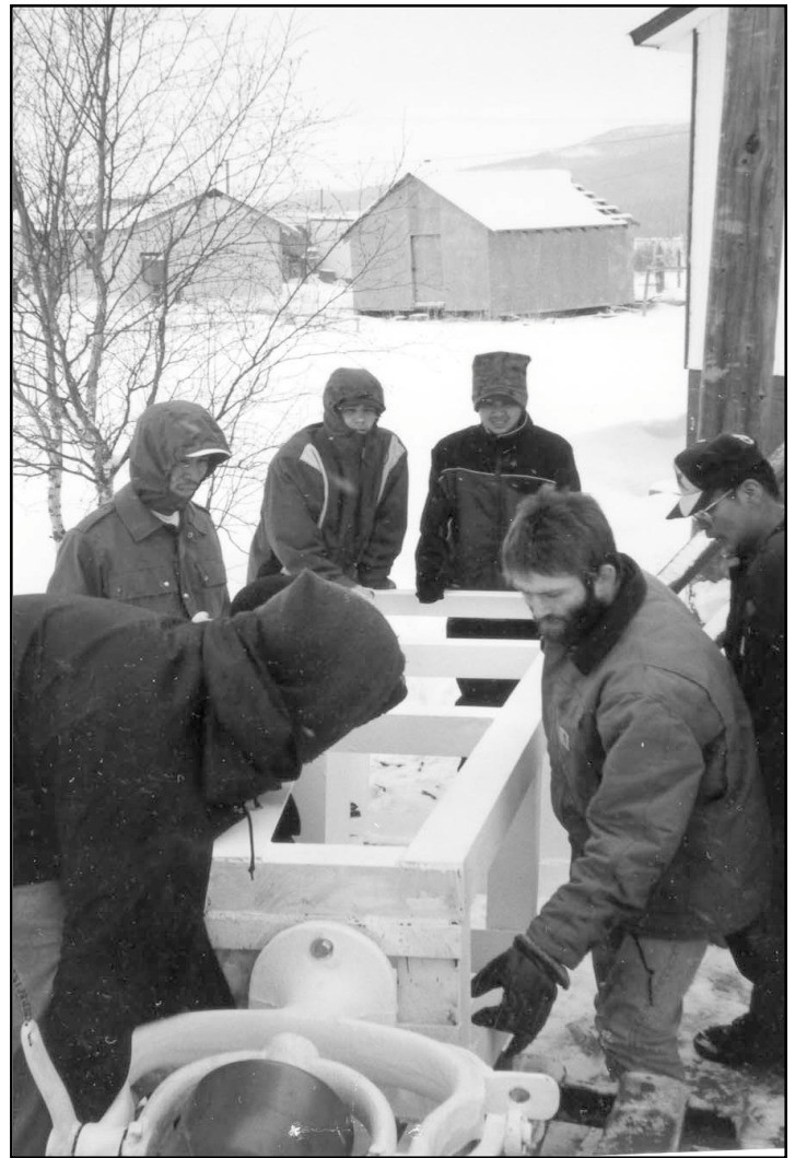
High schoolers, unload their new Bell tower that they constructed from leftover steel from the new church foundation.
